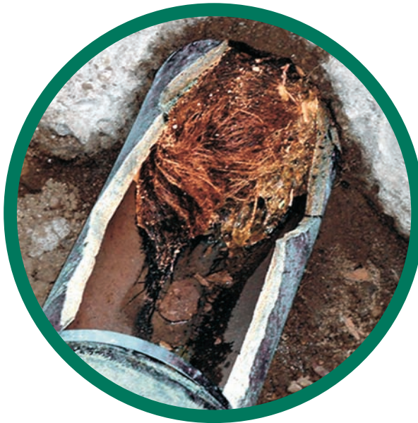
Photo shows tree roots that grew into a sanitary sewer line, caused a blockage and broke the pipe.
